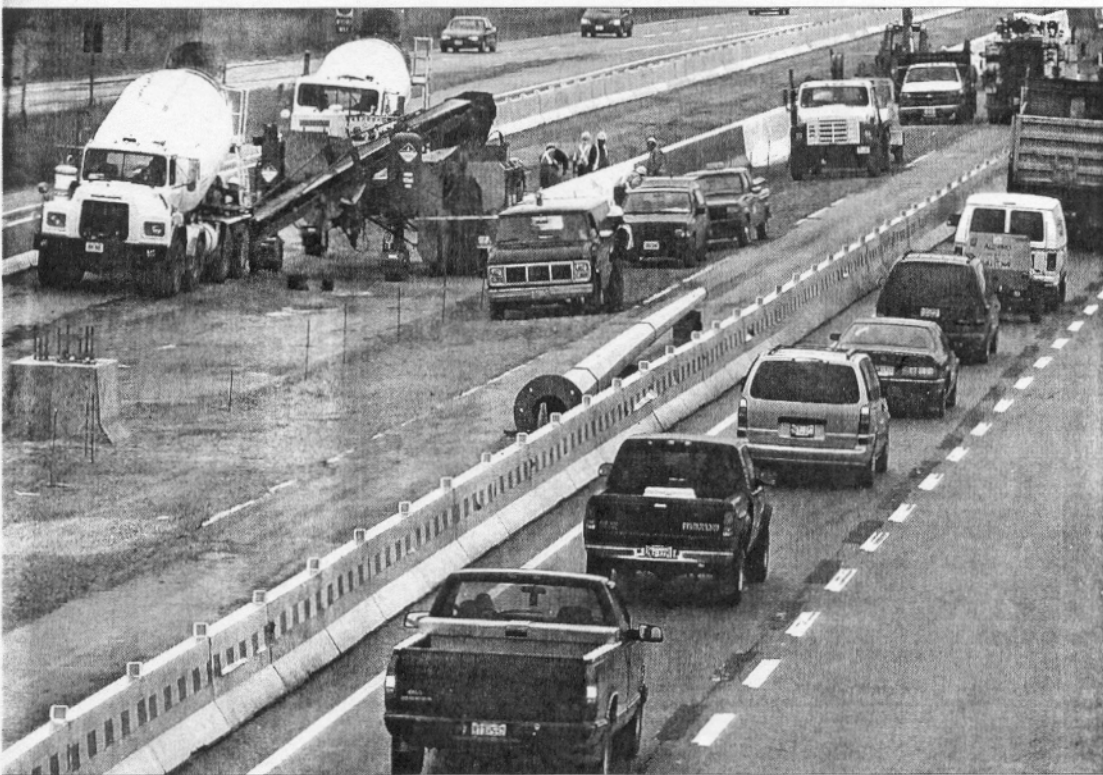
Highway construction along the Niagara Falls section of the QEW near McLeod Road recently.
